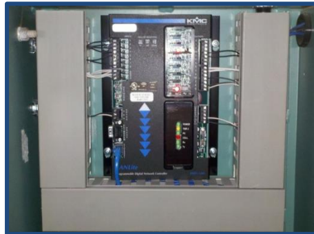
KMC Controls Before
