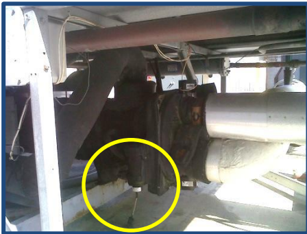
Level Sensor Before
