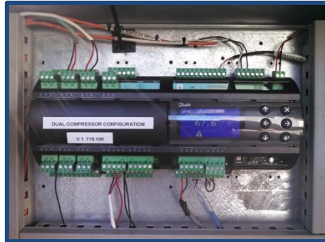
Danfoss Turbocor Controls After
